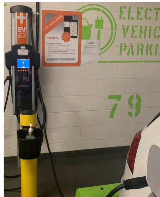
EV Charger, LDB Head Office
